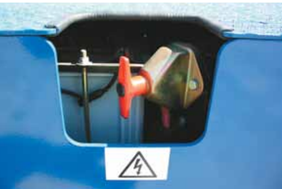
Emergency isolator switch is easy to reach at ground level
